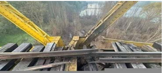
Ñuble region (Chile), June 13, 2023. The pulp industry’s railway bridge no longer functions
