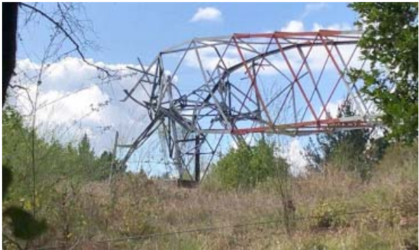
Los Álamos (Chile), June 9, 2023. The pylon of the high-voltage power line failed to withstand the shock of the attack.
