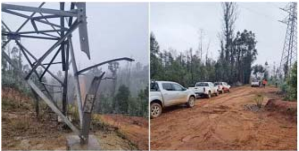
Placilla (Chile), June 9, 2023. The damaged pylon of the high-voltage line near Valparaíso.
